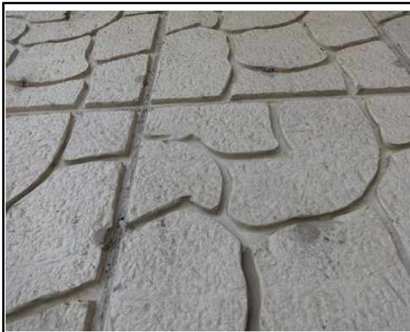
A1 균열 CW=0.2mm
